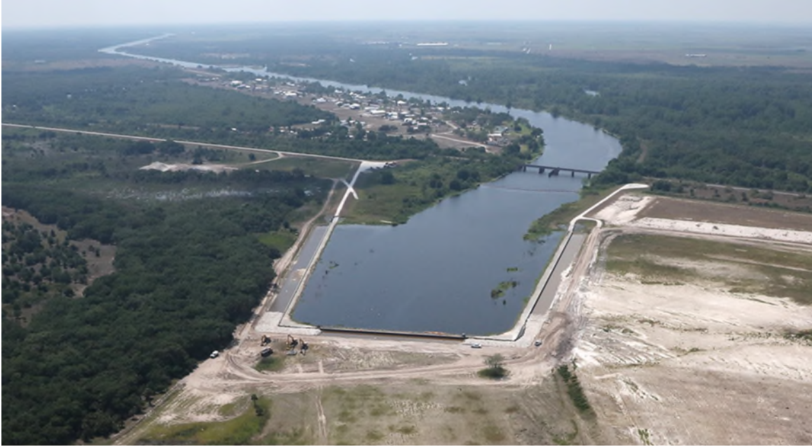
Figure 9-4. S-69 weir erosion repair and riprap installation post Hurricane Ian high discharges. (Photo by Brent Anderson in March 2023.)
