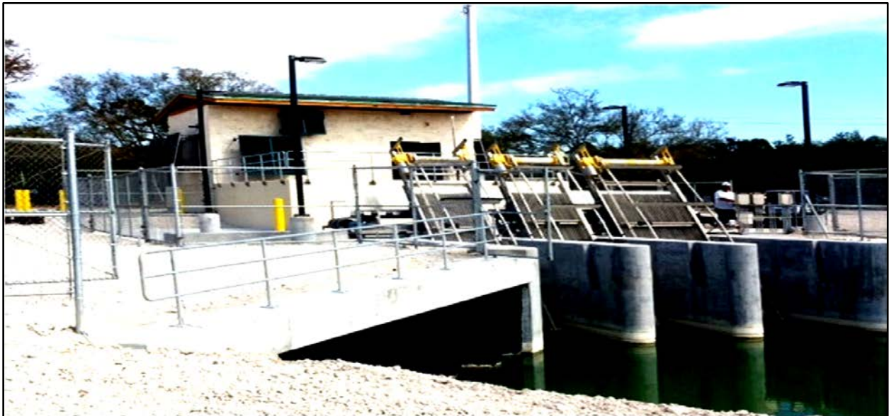
Figure A-4. Pump station S-700.
