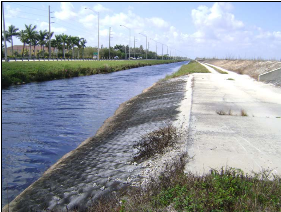
Figure 24. Closer view of the Emergency Spillway showing some vegetation growing along construction joints and fabriform joints.
