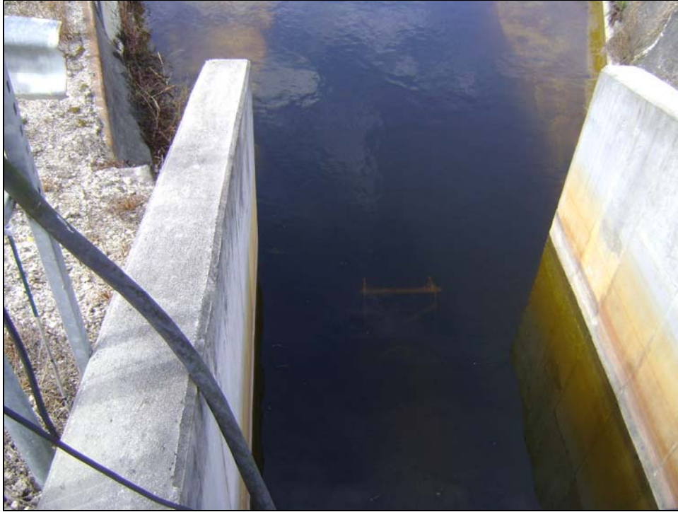
Figure 35. G-420S Seepage Pump discharge showing the flap gate.
