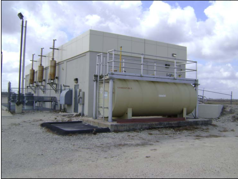
Figure 33. Southerly view of the G-420 Intake Pump Station showing the aboveground fuel storage tanks.
