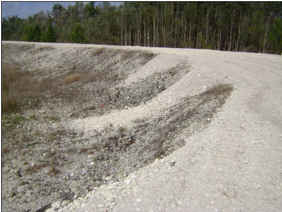
Figure 10. Northwesterly view of the northeast corner of the North Cell Perimeter Levee. The levee width is approximately 30- feet wide at this corner with the inside slopes at 0.75H:1V which will require flattening. Sparse vegetation on the slopes is withered. No ruts and erosion observed.
