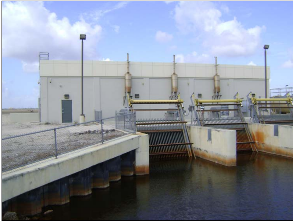
Figure 31. Westerly view of the G-420 Intake Pump Station showing the trash rake system and three pump bays with 223cfs electric pumps. The concrete abutments and steel sheet pile walls are in good condition.
