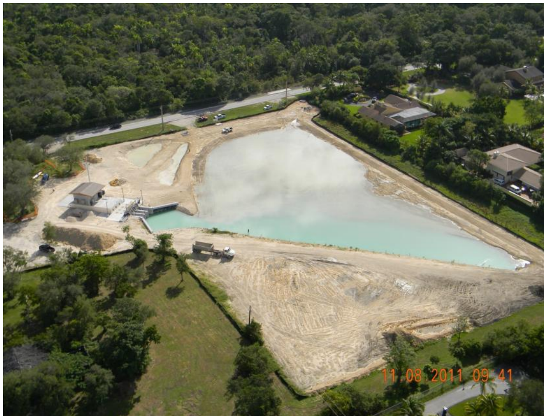
Figure 16- Biscayne Bay Coastal Wetlands, Deering Estate Flow-Way Pump Station (S-700)
