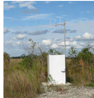
Figure 3. Groundwater well (photo by SFWMD).
