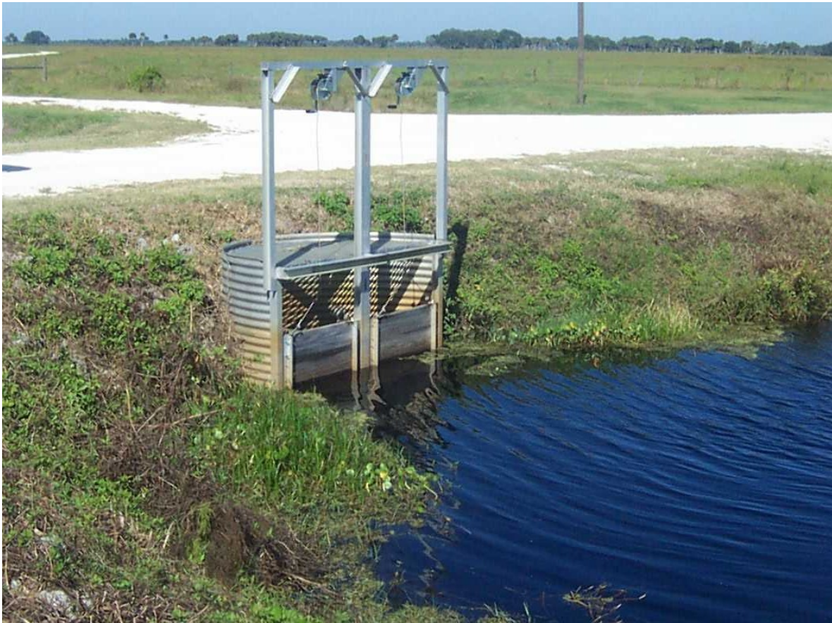
Figure 10-10. Example of an on-farm water management practice, specifically the use of a water control structure to retain storm water within on-site ditches. (SFWMD photograph).
